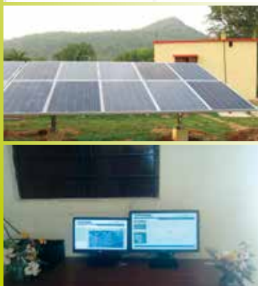
Picture 2: The village has been supplied with a 30 kWp Solar-powered Smart Nanogrid™ to meet the energy demands consuming about 20 kWp
