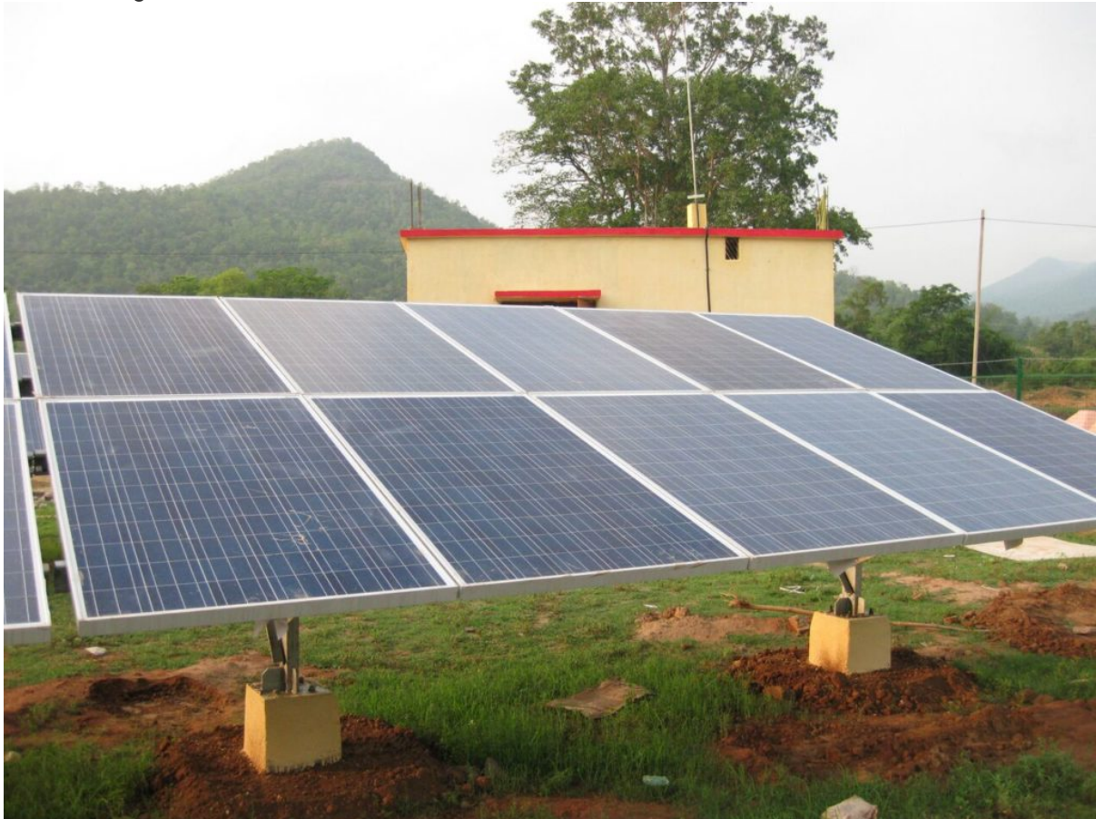
Solar panels in Chhotkei village
